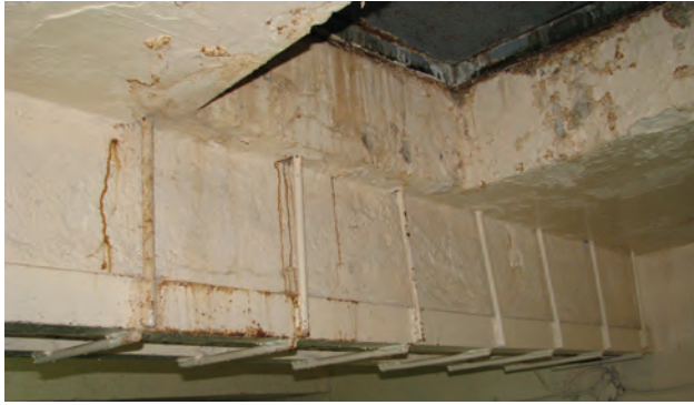
Fig. 2. View of corrosion of the floor and floor beams at the level of +4.20 in part B
