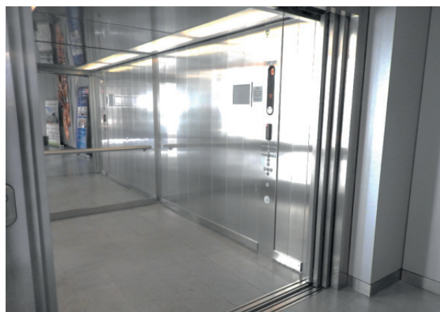
Fig. 28. Elevator in the building
